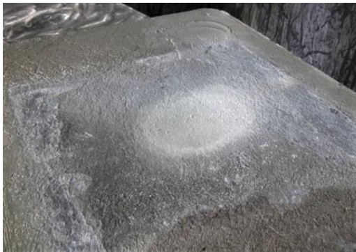
Excessive salt retention
