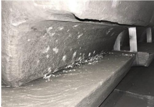
Heavy spots of localized corrosion
