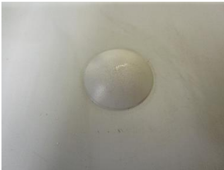
Photo No. 14 Typical Impact Dimple Detail (Interior)
